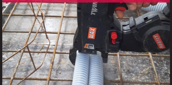
Electrical and plumbing piping
