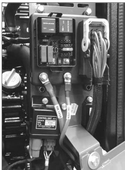
Fig. 256: Main fuse box
