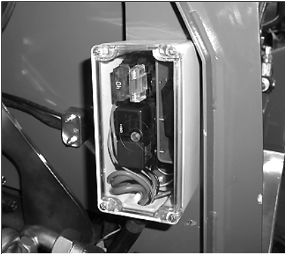
Fig. 190 : Main fuse box in engine compartment
