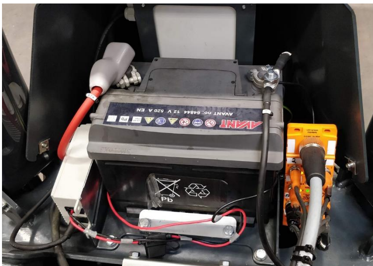
Figure 22 Battery is located in the back end of the chassis
