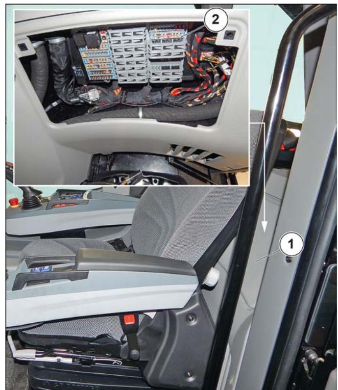
Figure 214: Fuse and relay in cab
