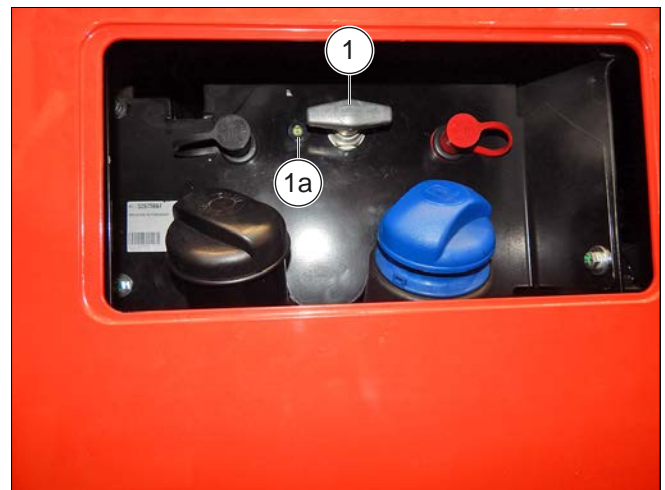
Figure 66: Battery disconnect switch
