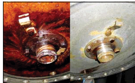
Vessel cover contaminated
